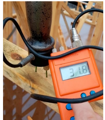
Wood with a moisture content of more than 25% can be damaged by moulds, fungi or insects.
