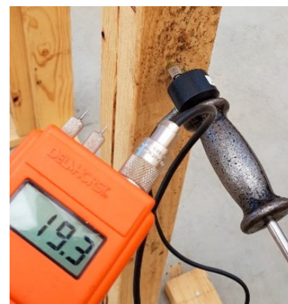
Wood with a moisture content of less than 20% can no longer support mould growth. MC should be less than 20% before any linings are installed
