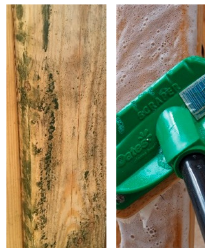
Normally, mould can be removed by washing the wood with a mild detergent and water.
