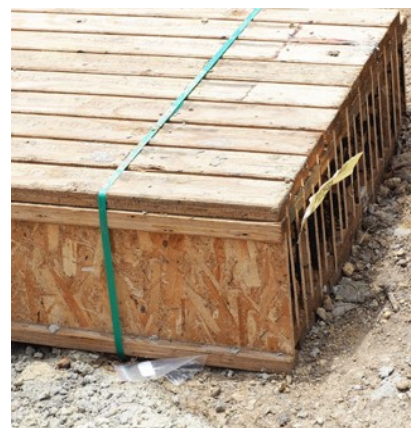
Timber should not be stored directly on the ground - use blocking or bearers to create separation.
