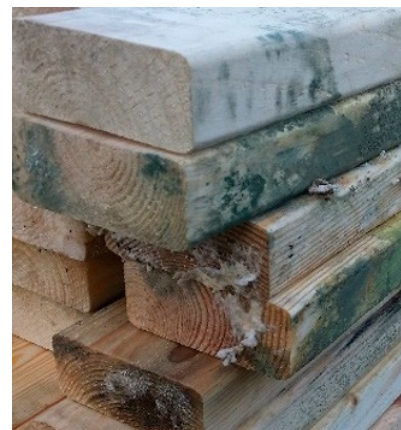
Mould growth on incorrectly stored wood looks bad but can be removed without lasting damage.
