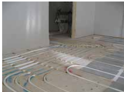
On-site milling for hydronic heating pipes at Limnologen Photo credit: Martinsons Byggsystem
