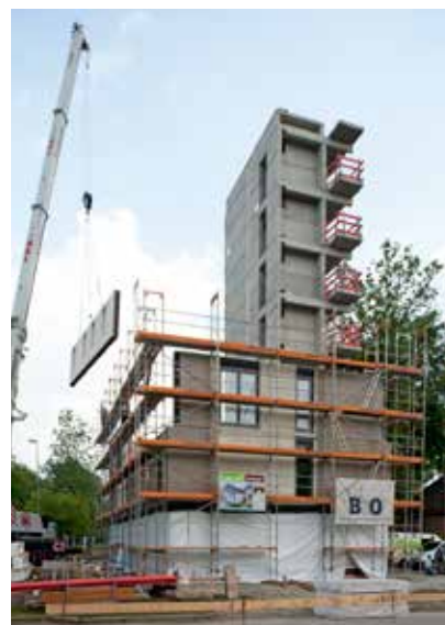
Prefabricated panel installation at Holz 8 Architecture by: Schankula Architekten Photo credit: Huber & Sohn
