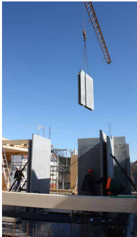
Installation of precast concrete element at 3XGRÜN Photo credit: Rozynski Sturm Architekten
