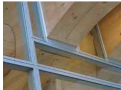
Notched interface conceals non-combustible barriers on timber beams at Tamedia. Architecture by: Shigeru Ban Photo credit: R. Holt
